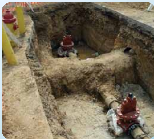
InsertValves on AC pipe for main control and hydrant replacement preventing asbestos fibers becoming airborne.
